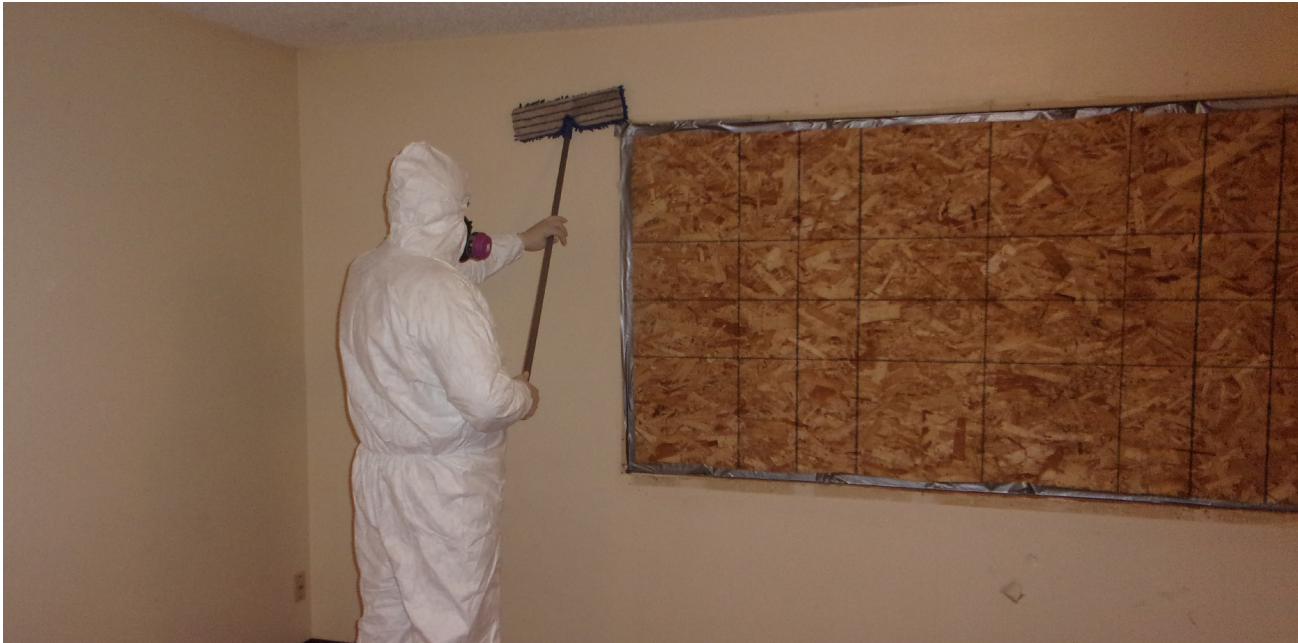
A certified remediation expert remediates a Salish & Kootenai Housing Authority unit contaminated by methamphetamine (Salish & Kootenai Housing Authority, 2021)
